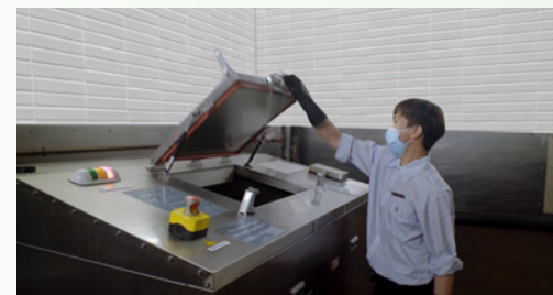
Onsite food waste decomposers were installed at Central Portfolio.
