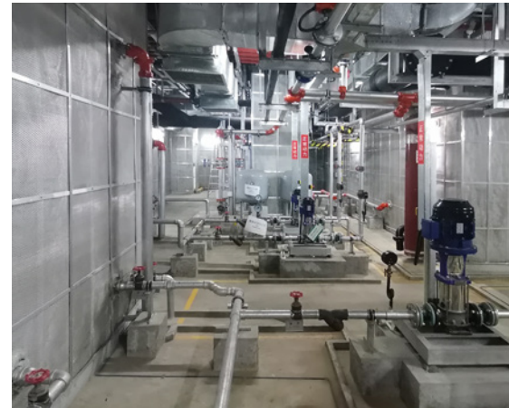
Our rainwater harvesting system at WF CENTRAL, Beijing.
