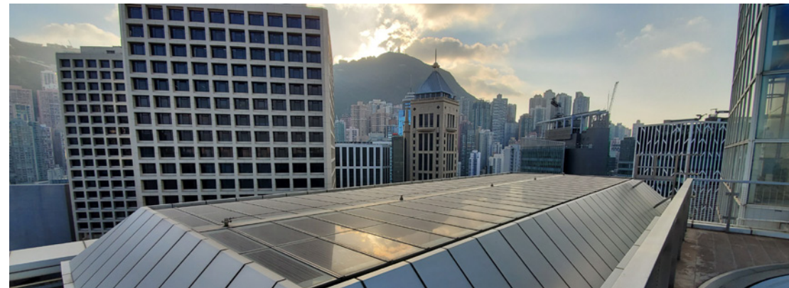
Solar Photovoltaic System at Chater House.
